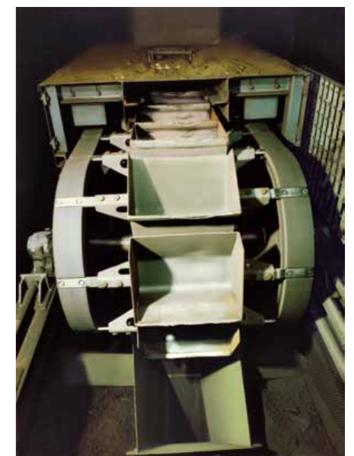
Belt and Pan Conveyor
