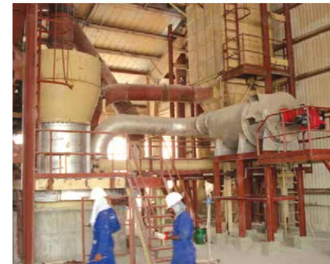
Roller Mills System with flash drying
